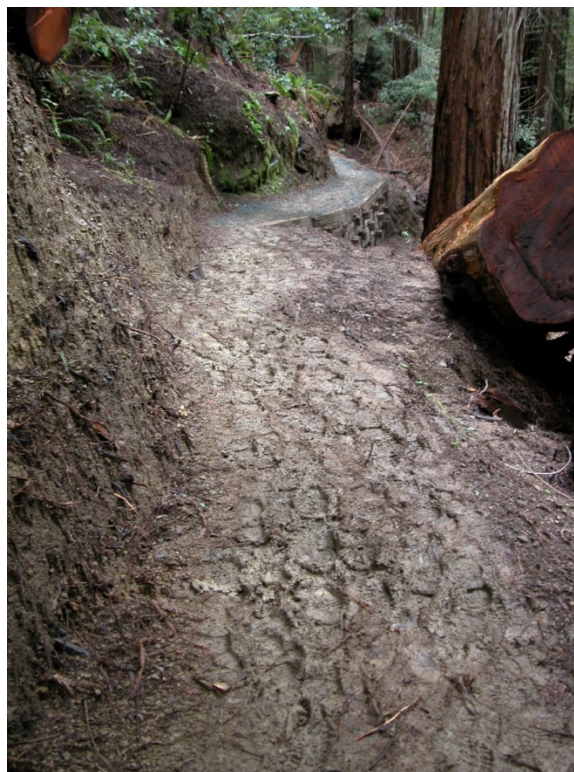
Photo 11.10 - Insufficient Trail Curing Resulting in Damaged Trail Surface
