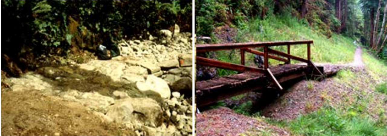
Photo 11.22 - Drainage Crossing Structures
